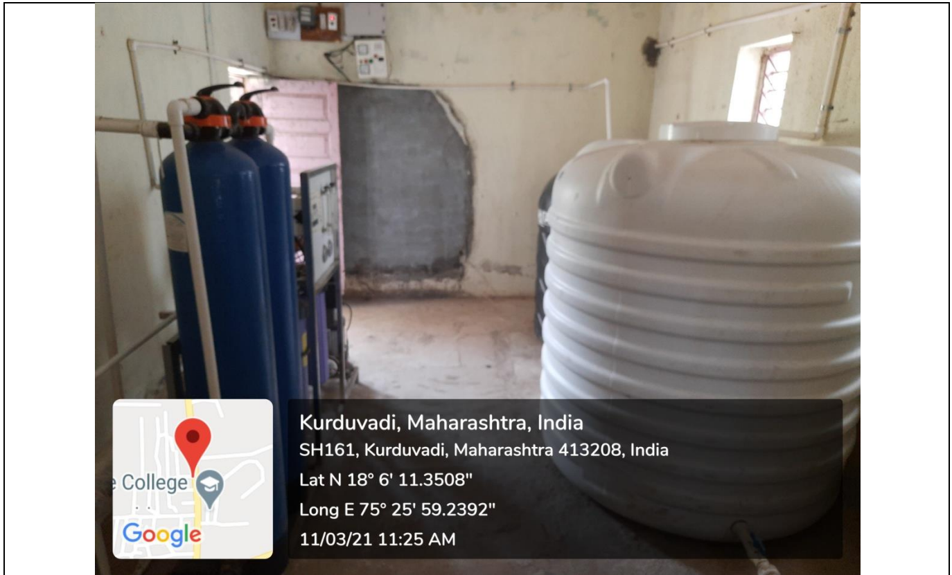
R.O. Water Plant
