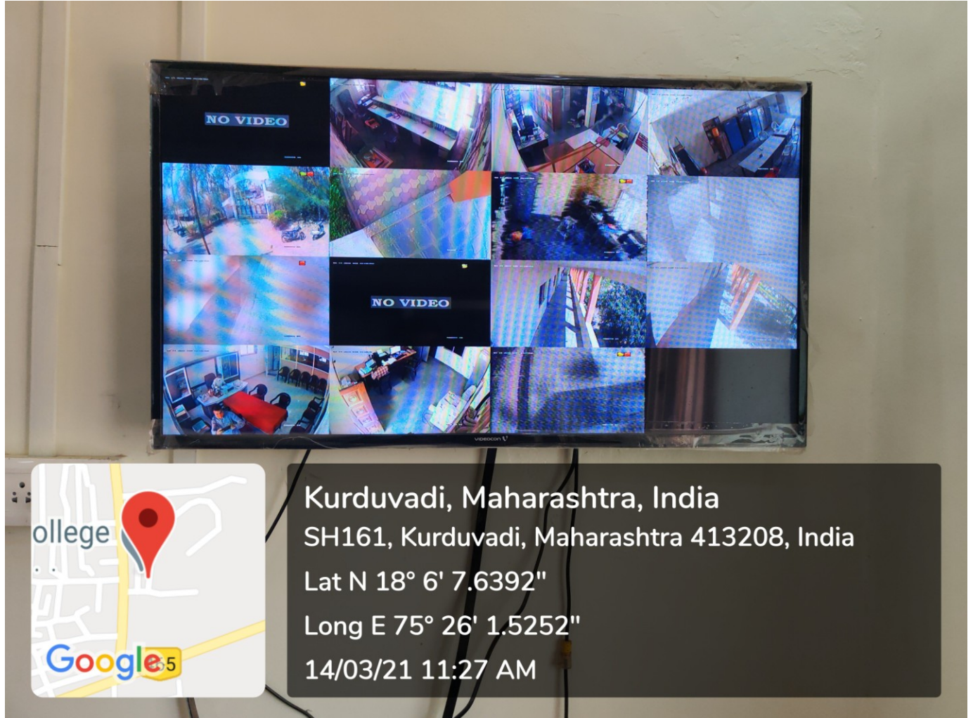
CCTV Coverage of Campus
